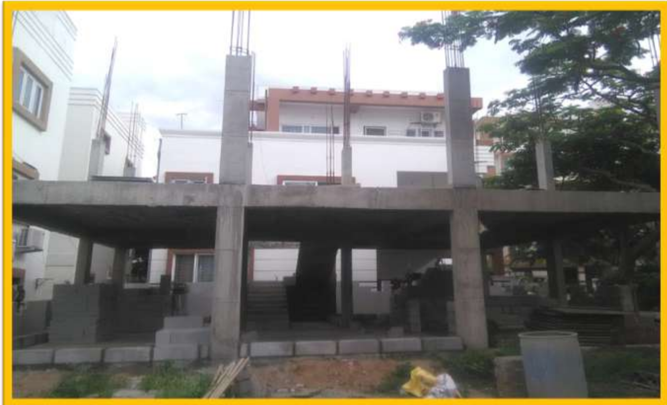
GROUND FLOOR SLAB AND 1 ST FLOOR COLUMNS CONCRETE & GR,FLR BRICK WORK IN PROGRESS.
