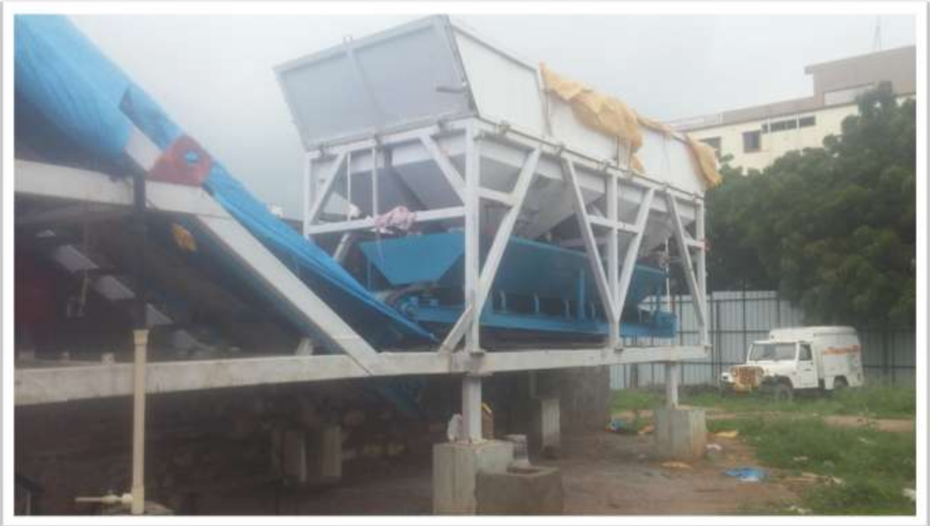
READY MIX CONCRETE MIXING BATCHING PLANT
